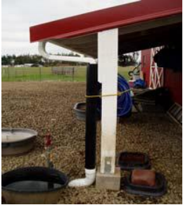
Downspout carries roof runoff to drywell.
