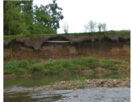
A streambank stripped of its natural protective vegetation and without any type of restoration is completely unprotected and highly erosive.
