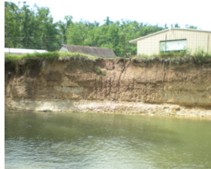
A highly unstable streambank has little to no vegetation and a vertical bank.
