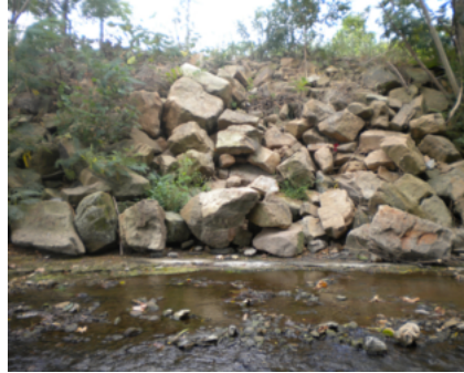
Riprap is an unsightly form of streambank protection that offers no pollutant filtration, wildlife habitat or aesthetics but can fix an unstable bank.
