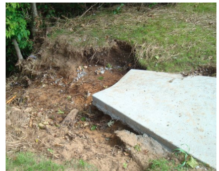
Runoff delivered to a creek by level spreader with no riprap protection or vegetative filter strip will deliver pollutants and become an erosion problem before entering a stream.
