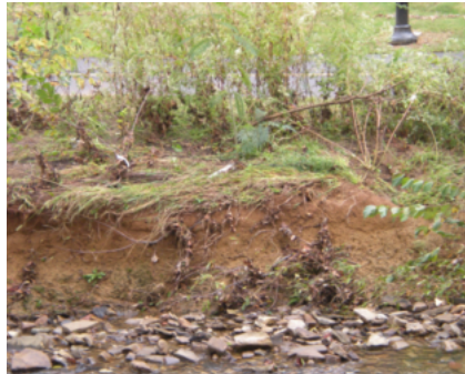
A moderately stable streambank has some vegetation and may or may not have a vertical bank.
