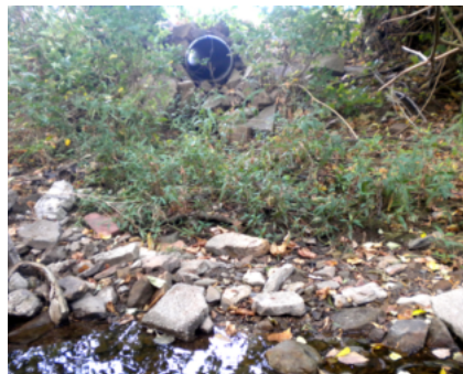
Drainage water delivered to a creek by pipe should have riprap protection around it and, if possible, should have to run through riparian vegetation before entering a stream.
