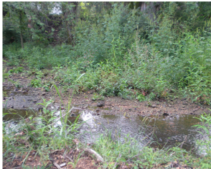
A stable streambank has a lot of dense and diverse vegetation and is usually not a vertical bank.
