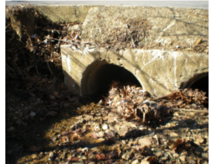
Culverts can clog with woody debris, trash and sediment. When this occurs, water flow can be blocked and aquatic wildlife movement can be limited.
