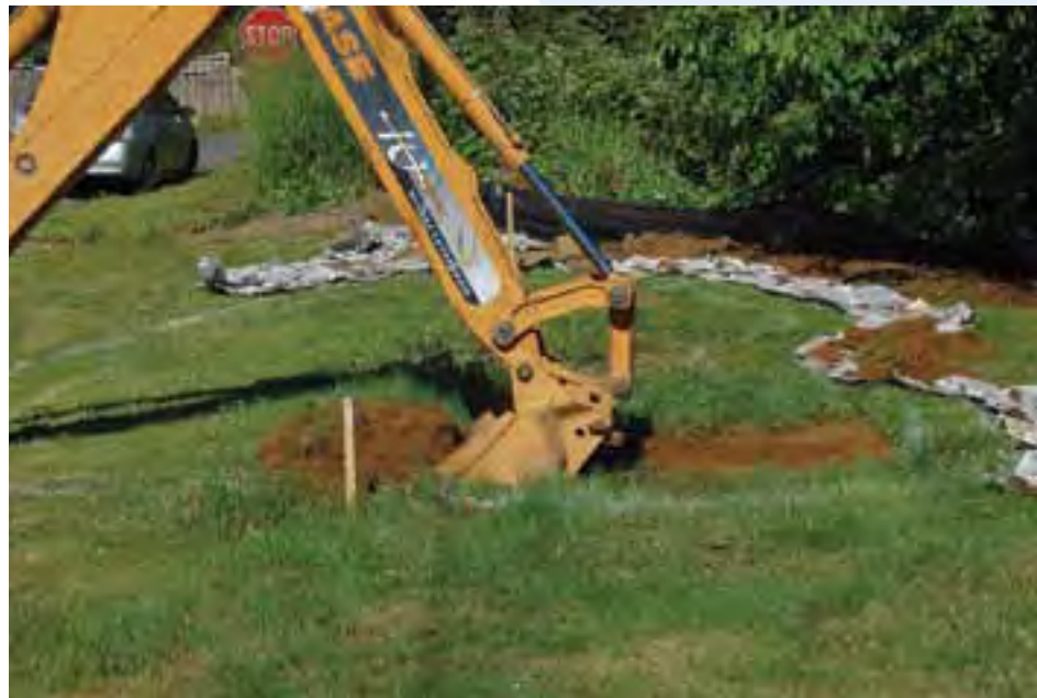
Figure 18: Excavator is located outside of the rain garden in order to make sure the machine does not compact soil in the rain garden. (Photo: Robert Emanuel, OSU)
