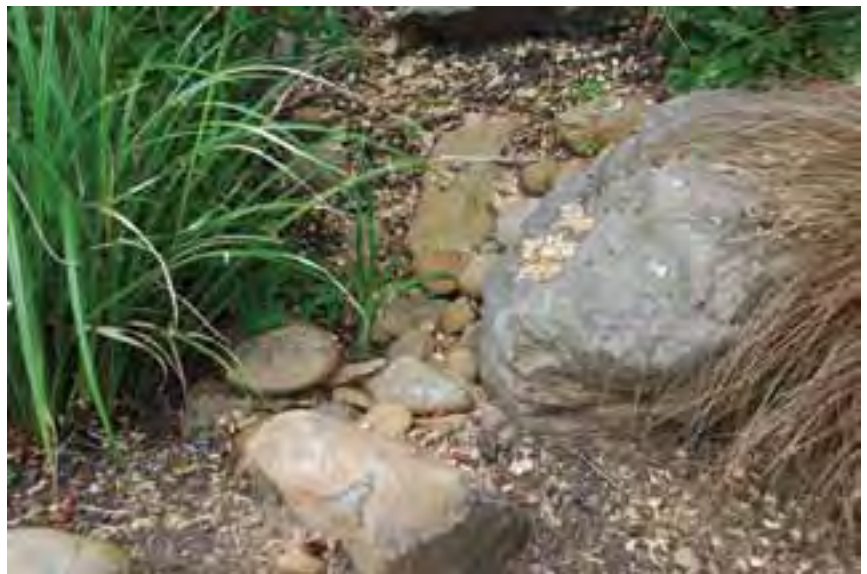
Figure 24: An outflow notch in a Portland, Oregon, rain garden, protected by rock to prevent soil erosion. (Photo: Robert Emanuel, OSU)
