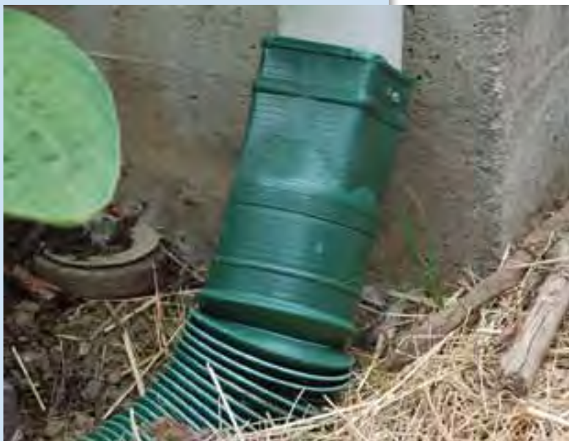
Figure 14. Downspout connected to downspout extension that directs flow away from a building's foundation. Note sheet-metal screws. (Photo: Robert Emanuel, OSU)
